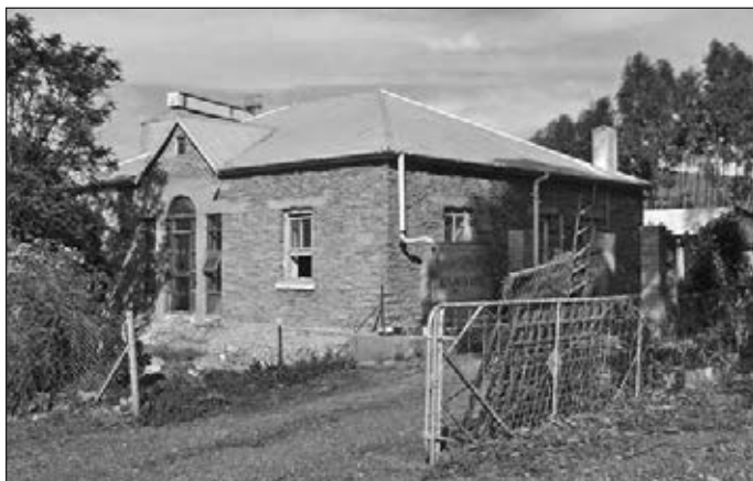
Below: The front of the building with plaster removed and exposing the leiklip construction, common in the village and surrounds.
