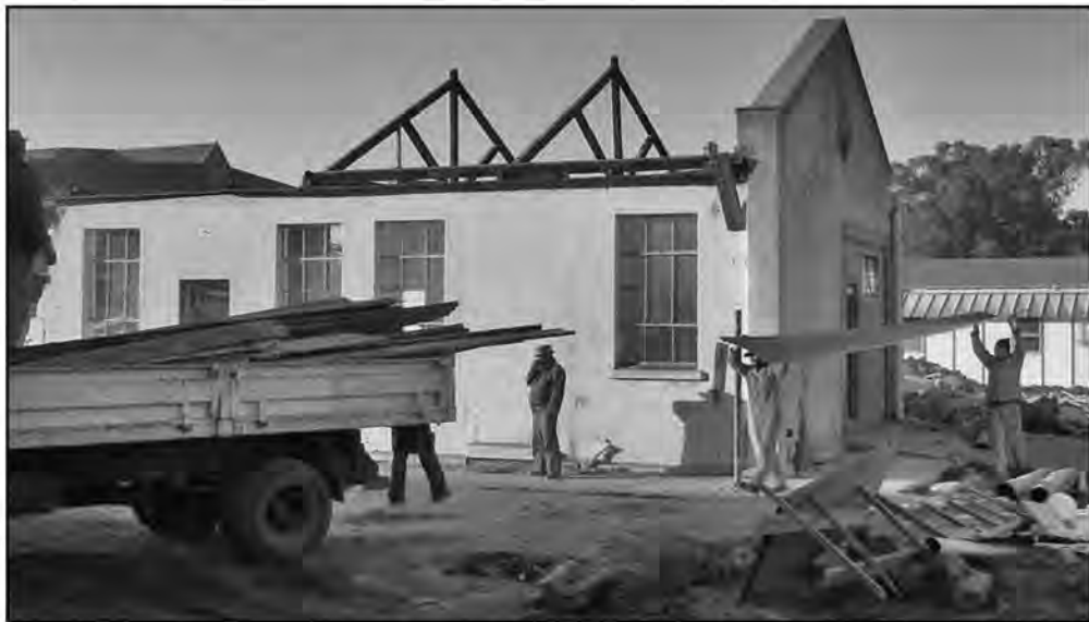
Re-usable materials being removed from the site of the old power station
